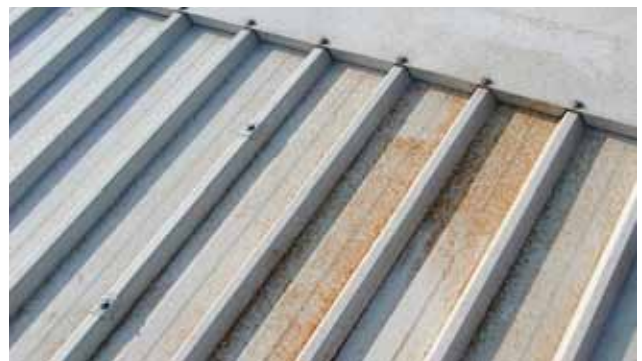
Picture 34. View of lacquer coating damaged by filings during cutting with an angle grinder
