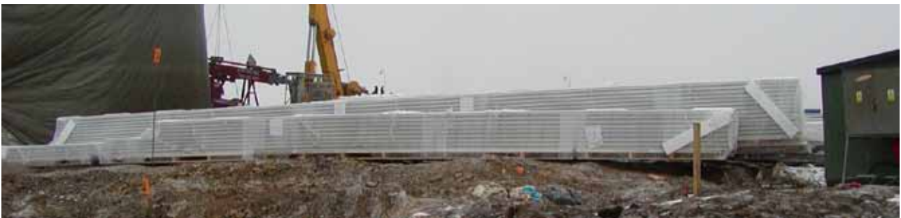
Picture 9. Panels stored incorrectly
