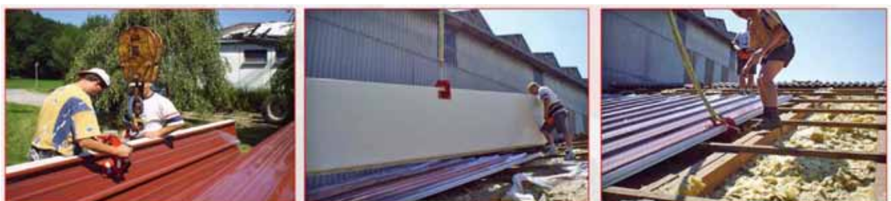
Picture 26. Stages of transportation of roof panels with the help of a self-locking assembly tool.
