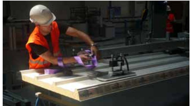
Picture 22. A sandwich panel turned over on columns.
