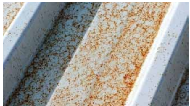
Picture 35. Damage to lacquer coating caused by leftover rusted filings
