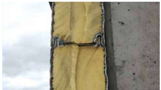
Picture 33. View of burnt panel cut with an angle grinder.
