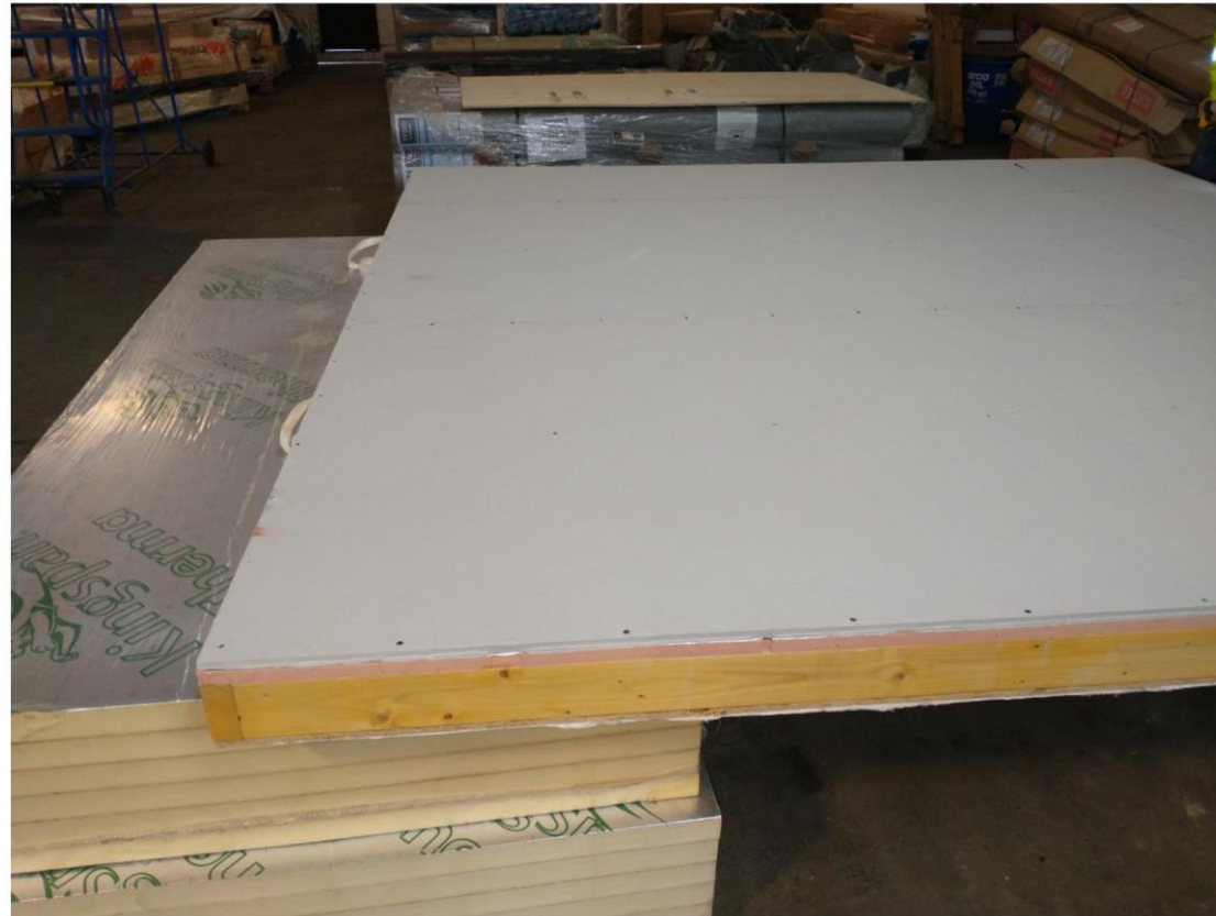
Photograph 5 – View of the completed sample, prior to applying tape and jointing compound
